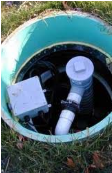
Typical NEMA 4 junction box for pump tank. A better installation would be to run the wires through the riser and mount the box externally.
