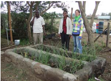
Greywater system for Crater Secondary School (Nakuru, Kenya) implemented by the ROSA project. Photo courtesy Sustainable Sanitation's Photostream ( www.SuSana.org )
