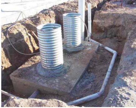
Outdoor commercial grease interceptor. Note that sanitary wastewater is routed to bypass the interceptor to keep grease clean for reuse or recycling.
